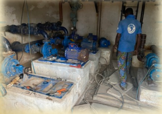
Utilities Pump Room in mango
